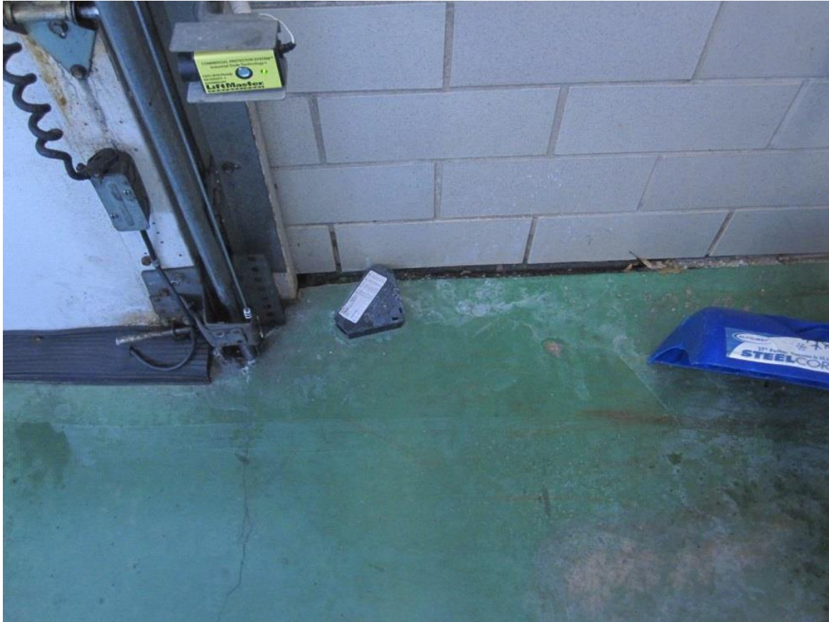
ARCHITECTURAL PICTURE 1: Floor settlement at south wall. No visible floor or wall cracking.
