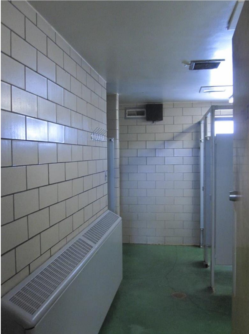
ARCHITECTURAL PICTURE 2: Limited space in restroom. All interior walls concrete masonry and glazed block.
