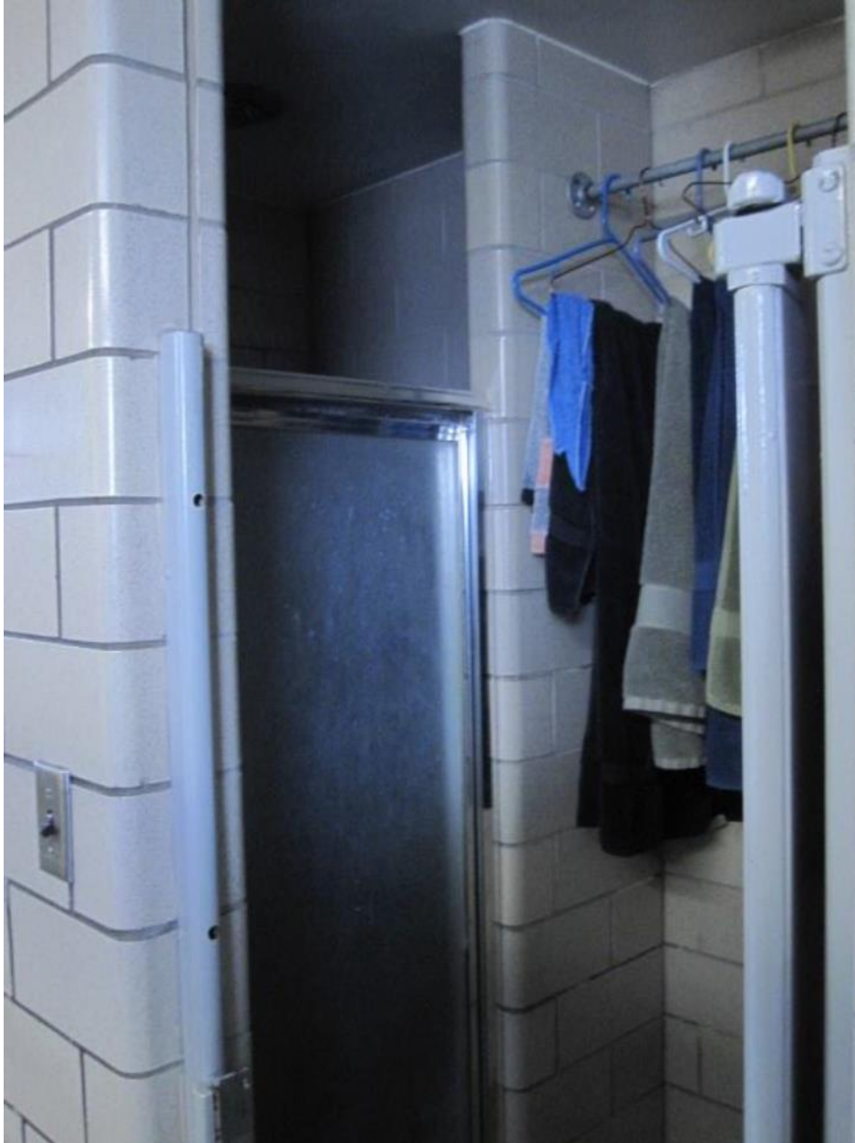
ARCHITECTURAL PICTURE 3: Narrow shower clearances not compliant with ADA/ANSI codes.
